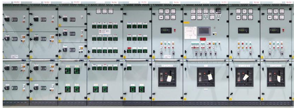
690V Main Switchboard with ABB Breaker
